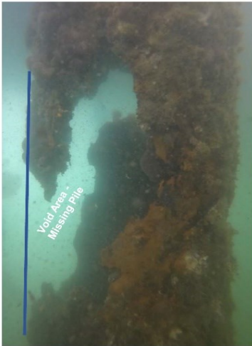
Figure 2 Figure 2 Example of batter pile with corrosion to point of perforation (Echelon 2021).
