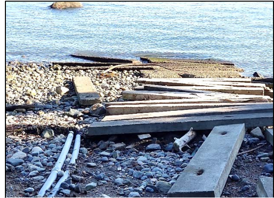
Photo 2. Derelict concrete plank boat ramp (Herrera, Sept. 30, 2019)
